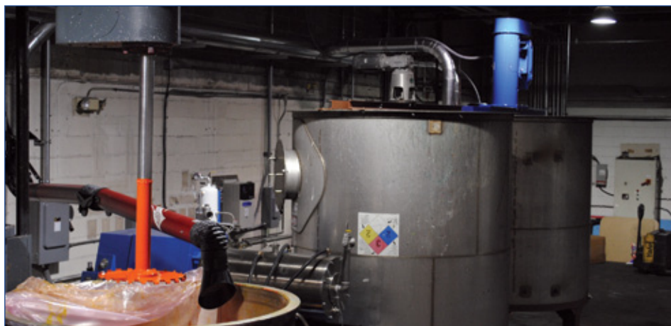
Toll milling at Custom Milling & Consulting
