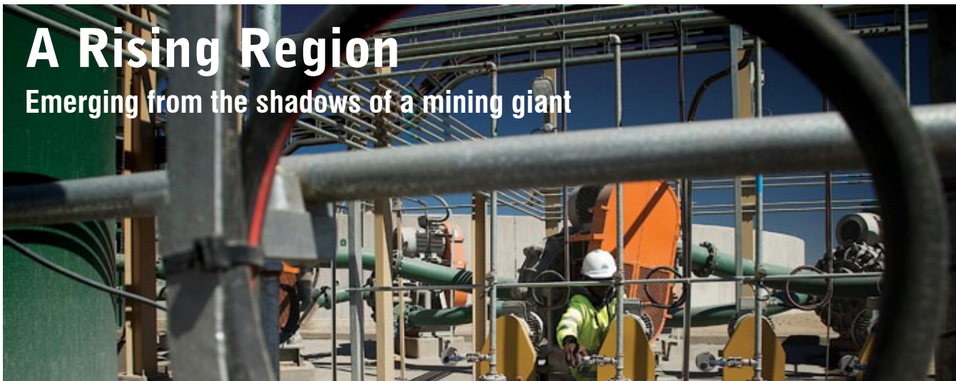
Skilled (Trained) operator checking the pressure on the gland water pumping system. Photo courtesy of Minopex.
