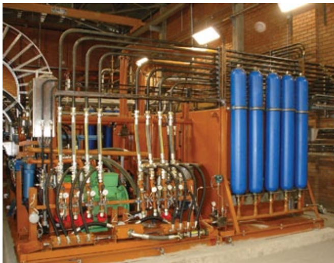
9,000 litre hydrostatic oil circulation system, designed, manufactured and installed by OMSA. Photo courtesy of OMSA.
